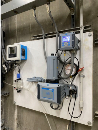
Turbidimeter at WTP
