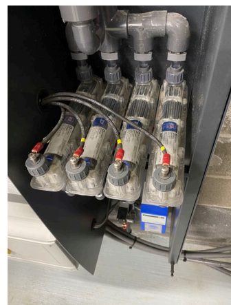
Cells for OSG at WTP
